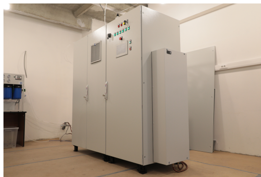
Electrolyzer for hydrogen production
